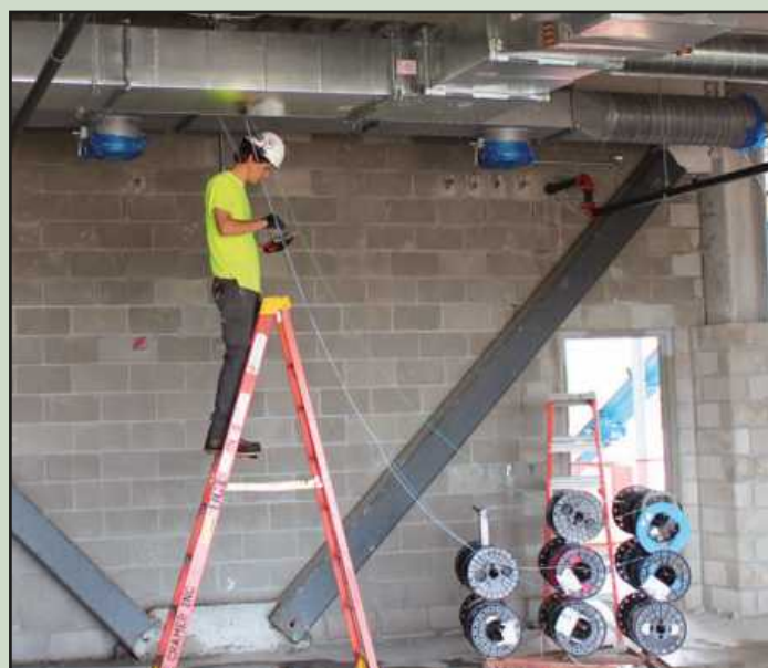
PULLING WIRE at the Saginaw United High School project is apprentice Matthew Riebschleger of IBEW Local 557. He's employed by Thiel Electric.
