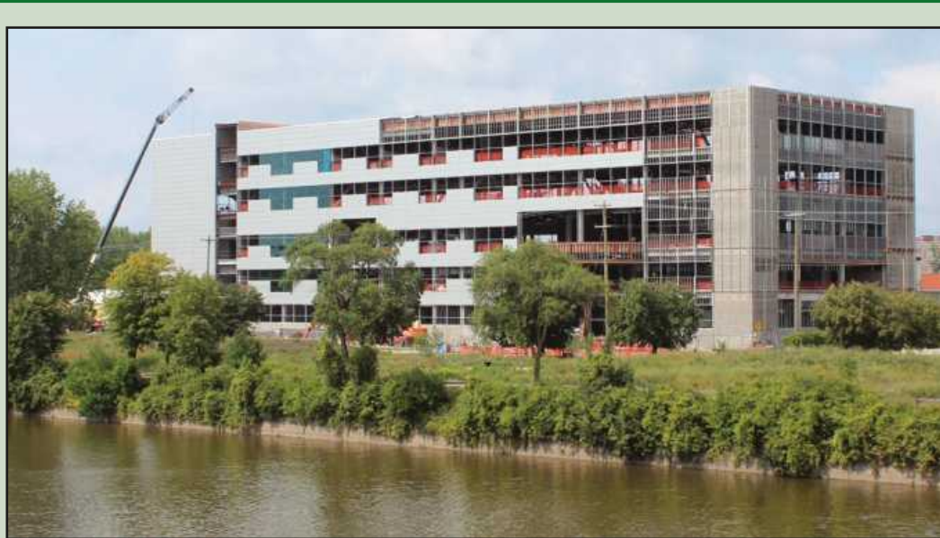
IT HAS BEEN AT LEAST 80 years since Saginaw high school students have been able to learn in a new building. That will change next year with the opening of the new Saginaw United High School, shown under construction on the Saginaw River.
