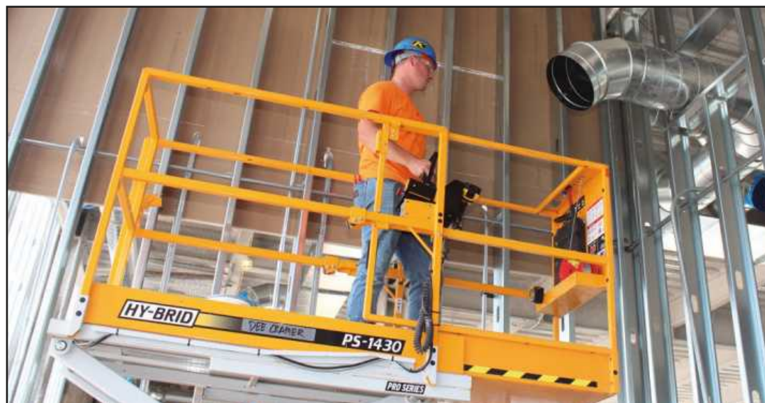
SETTING DUCT WORK at Saginaw United High School project is Tom Fortney of Sheet Metal Workers Local 7. He's employed by Dee Cramer.
