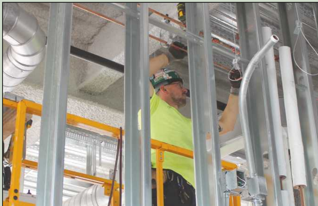
SETTING DOMESTIC water lines at the Saginaw United High School project is Ryan Mulka of Plumbers and Steamfitters Local 85. He's employed by Johnson and Wood.
